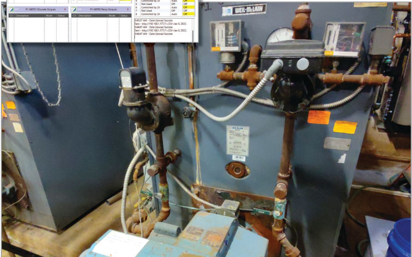
Figure 3. Typical HVAC systems use many types of equipment and packaged systems, which must be directly controlled or supervised to deliver the proper environmental control and utilities.
