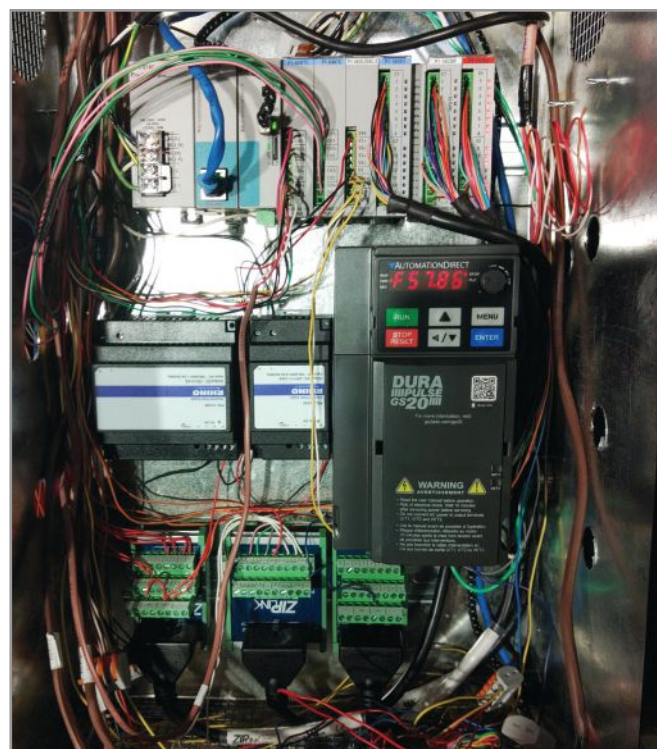
Figure 2. HVAC projects need to monitor temperature, humidity, pressure, and airflow sensors, and control solenoids and valves. In some locations, variable speed drives were needed for fan and pump control.
