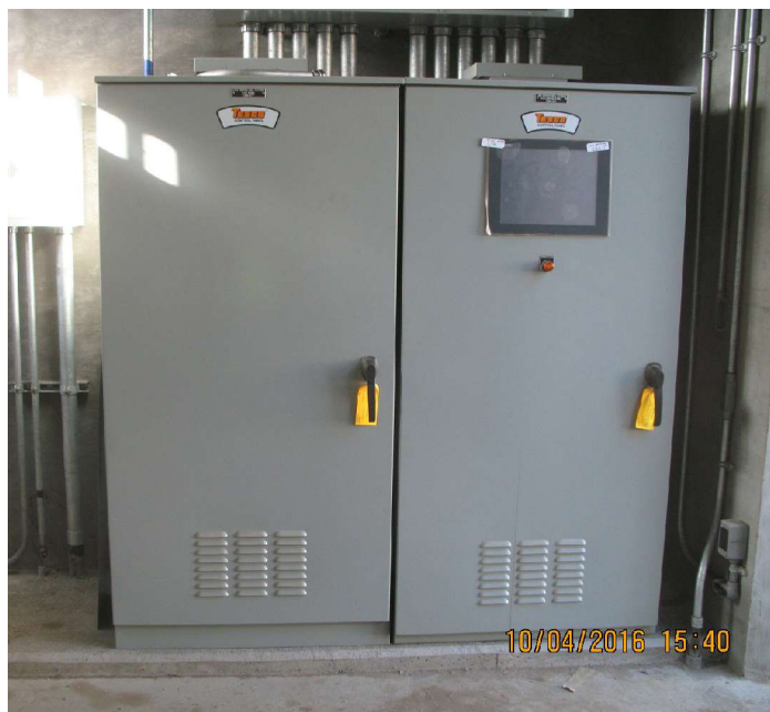
Figure 4. Lake Merced PLC master controller. The PLC is a redundant CPU with hot backup connected to AVPN network with redundant fiber-optic cables.
